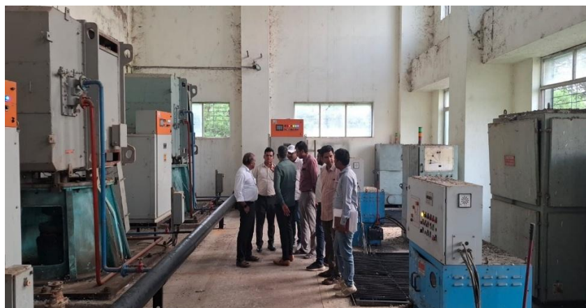
Mhaisal Pumphouse Stage No.5, Salgare
