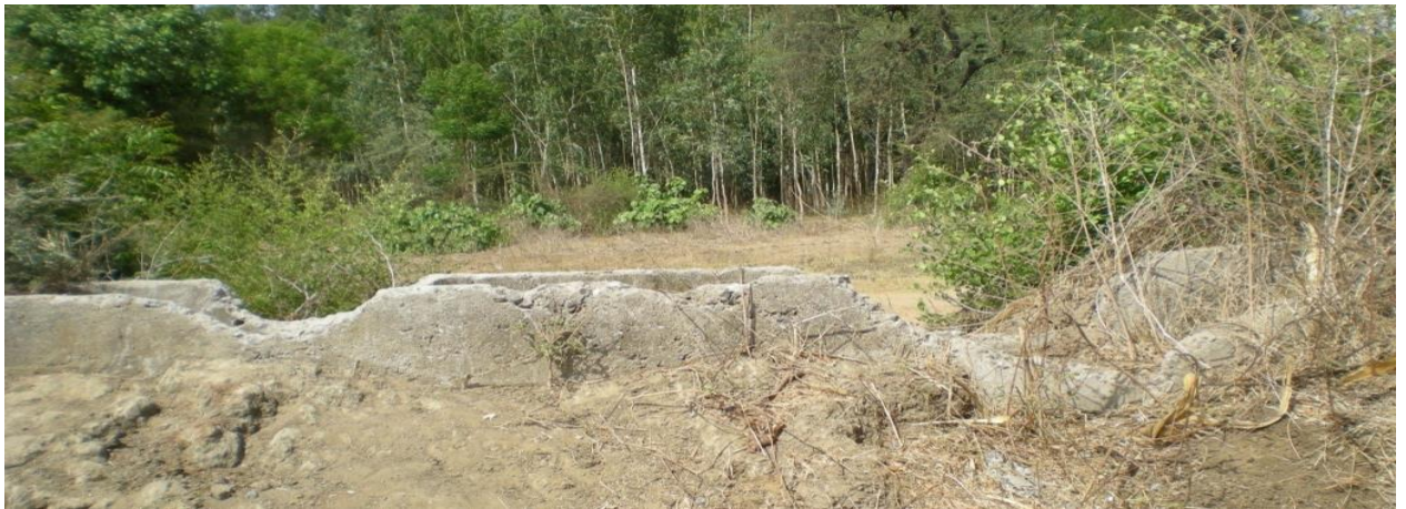
Damaged Open Gravity channel
